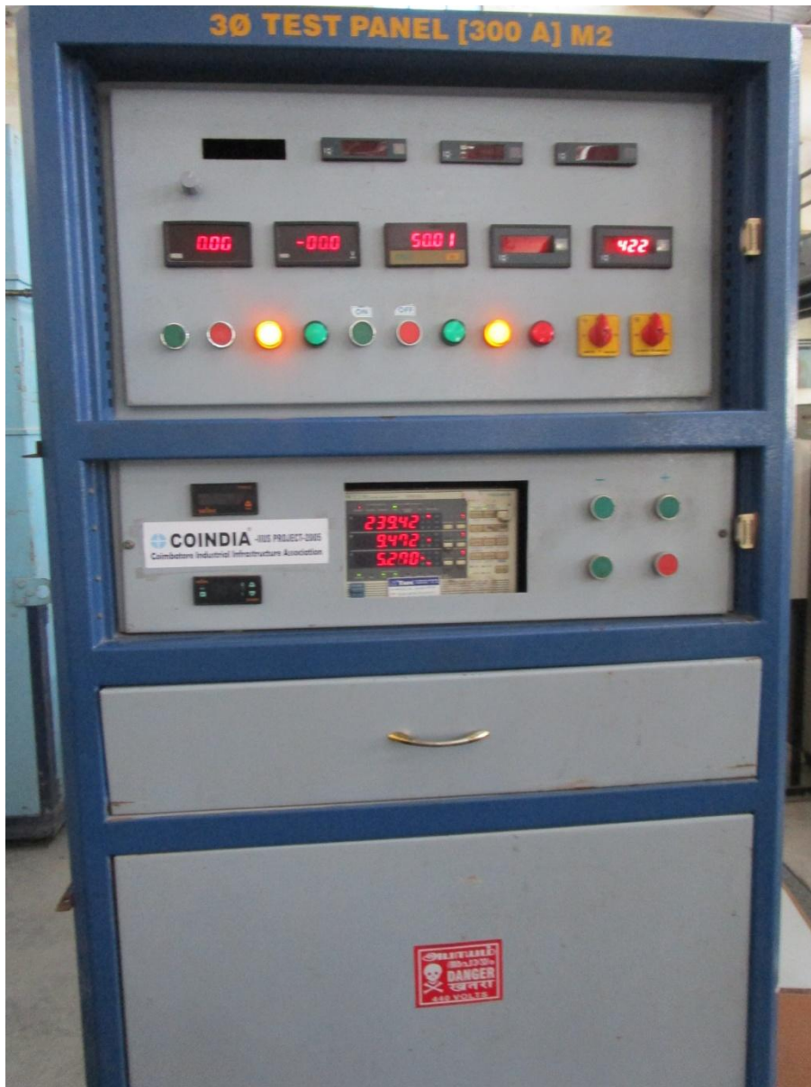
Figure 3.5(b) Three phase AC control panel for power measurement
