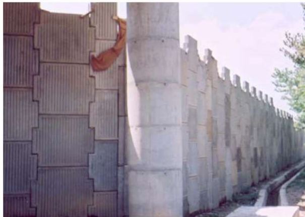
Fig. 3. (Top) Damage sustained by buildings in Uri 30 km from site and (Bottom) MSE approach wall for Bridge No. 127 after the earthquake [5].
