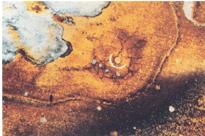
e) Extensive corrosion under the residue and in cracks in the residue: Major Corrosion
