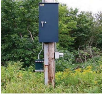
Fig. 5 a Pad Mounted Service Cabinet
