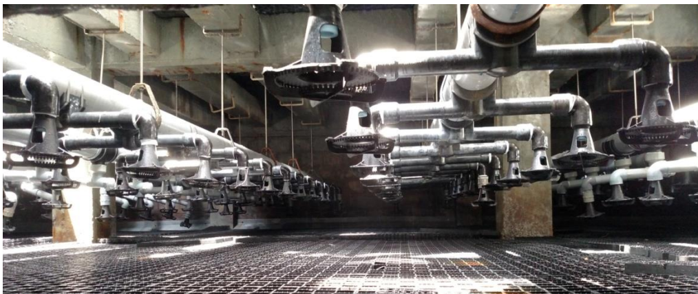
(Arrangement shown is indicative and may vary in practice) FIG. 9 DISTRIBUTION PIPES FIXED BELOW RCC BEAMS
