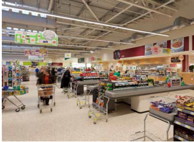
Fig. 23 Cashier And Checkout Area Lighting
