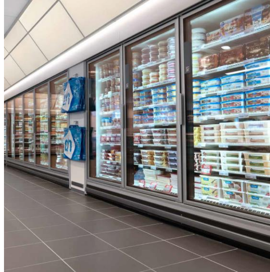
Fig. 22 Freezers and Coolers Lighting
