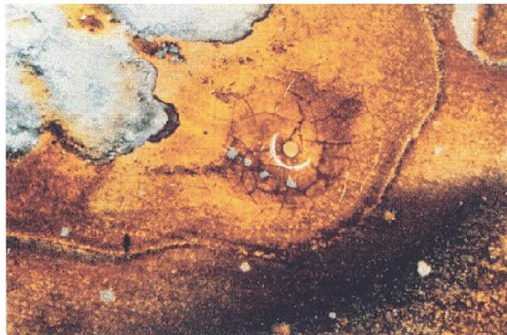
e) Extensive corrosion under the residue and in cracks in the residue: Major Corrosion
