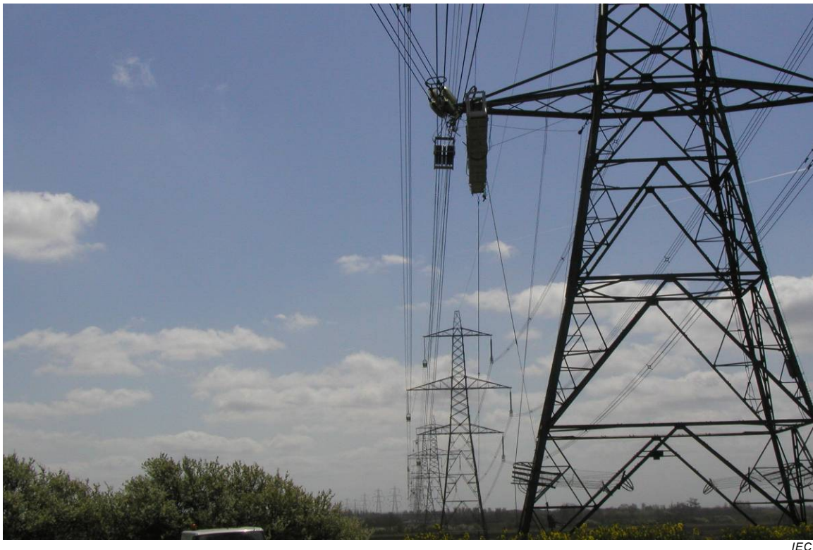
m) Transmission – Reconductoring operation on double circuit power line with one circuit live
