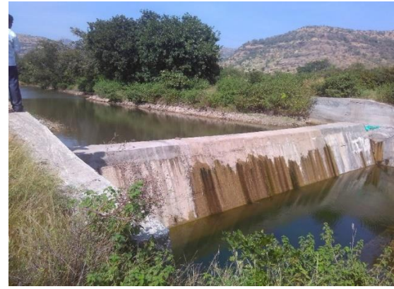
FIG. 7 PHOTOGRAPHIC VIEW OF A TYPICAL NALLAH BUND
