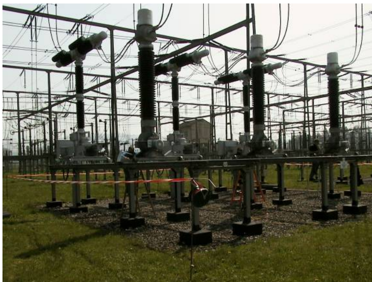
a) the 245 kV part of the substation GM Mettlen/CH
