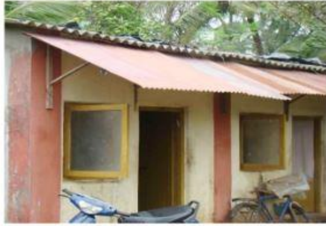
FIG. 12 MASONRY EXTERNAL WALLS AND A TIMBER FRAMED UN-TRUSSED LEAN-TO-ROOF WITH AC AND GI SHEETS
