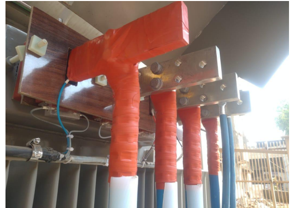
Bus Bar Insulation
